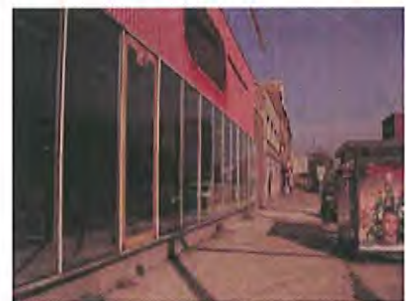
Many storefronts in the area, however, require maintenance. Also, sidewalks are cracked, full of weeds, and in need of repair.
