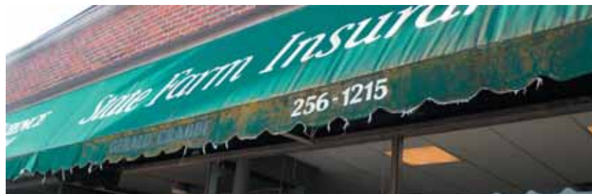
Awnings on several buildings are in need of replacement.
