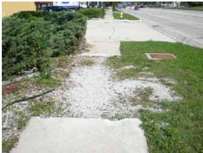
Missing sidewalk on west side of La Grange Road near 144 th Street
