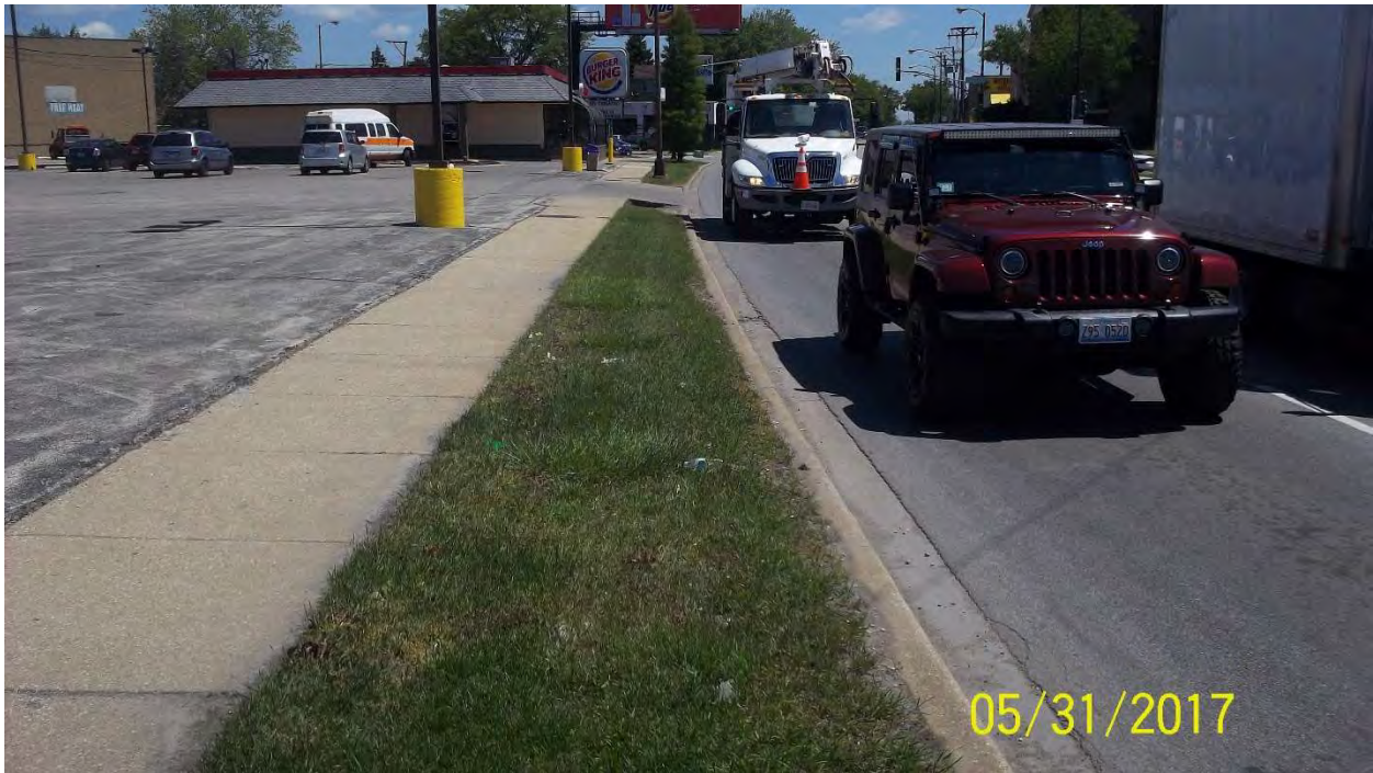
Photo 58: Northwest corner of 79 th St. / Columbus Ave. East of Sawyer St.– Looking Northeast
